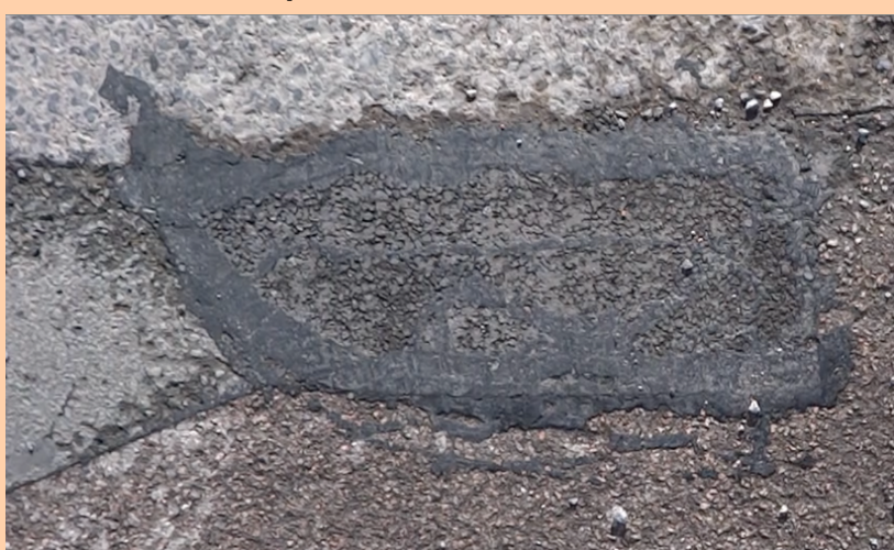
'A patchwork of tar'
